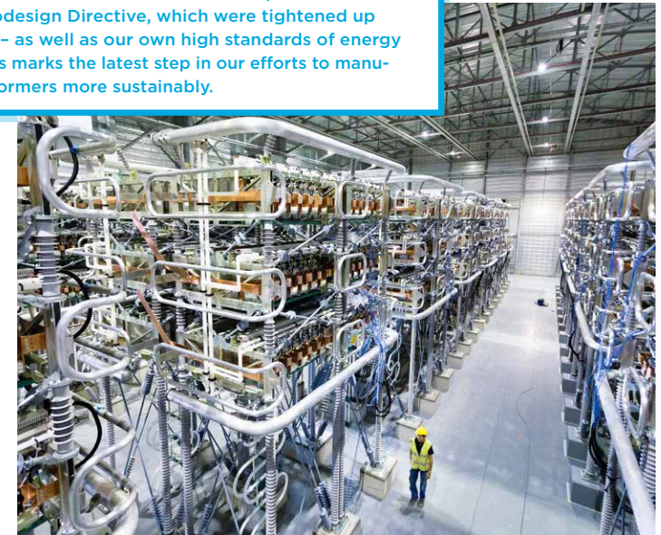
Amprion is procuring more climate-friendly electrical steel strips comprised of core laminations for the A-Nord and Ultranet converter stations.
