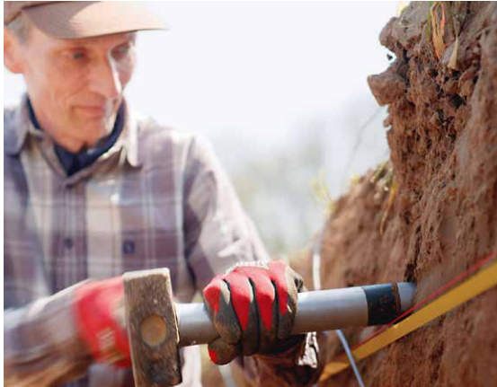
The ALEGrO line uses HVDC transmission technology and was installed as an underground cable.
